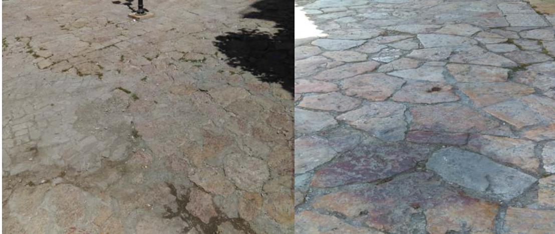
Figure 1 Current situation of (damaged) pavement and pavement in good condition
